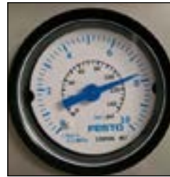
Sufficient pressure >5 bar
