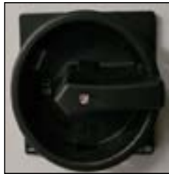
Main switch off
