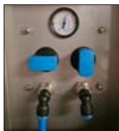
Connection on compressor
