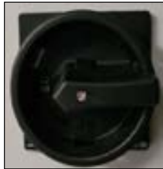
Main switch off
