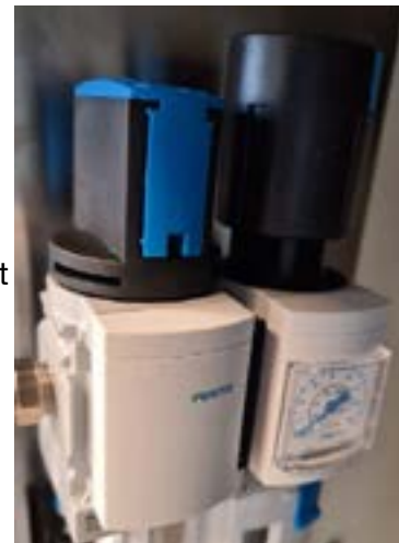
Shut-off valve compressed air in closed position
